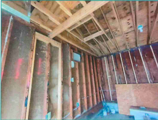
Repairs in garage for prior fire damage. Water staining throughout garage tested dry.
