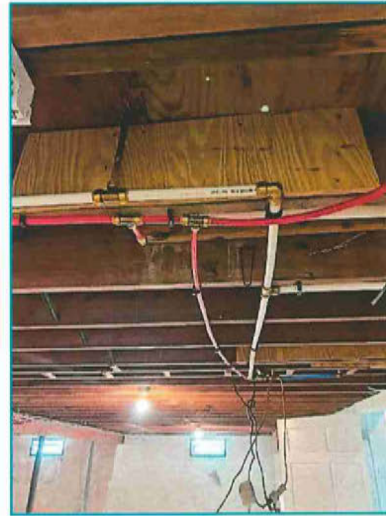
Repairs to previously damaged / notched joists in basement (3/6/2024). Repairs appear to adequately address prior damage.
