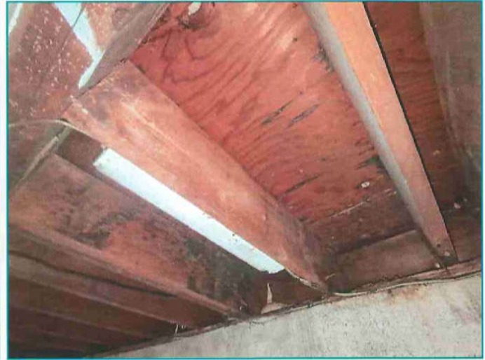
Water staining with elevated moisture below front door.
