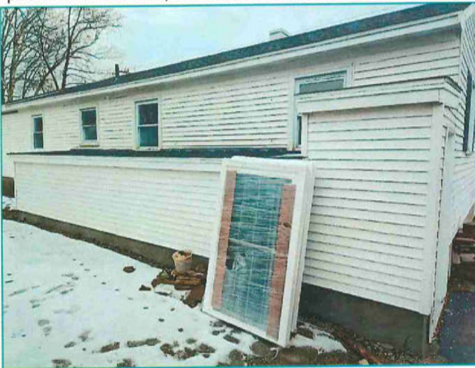
Roof is leaking / wet conditions at interior of basement entry.
