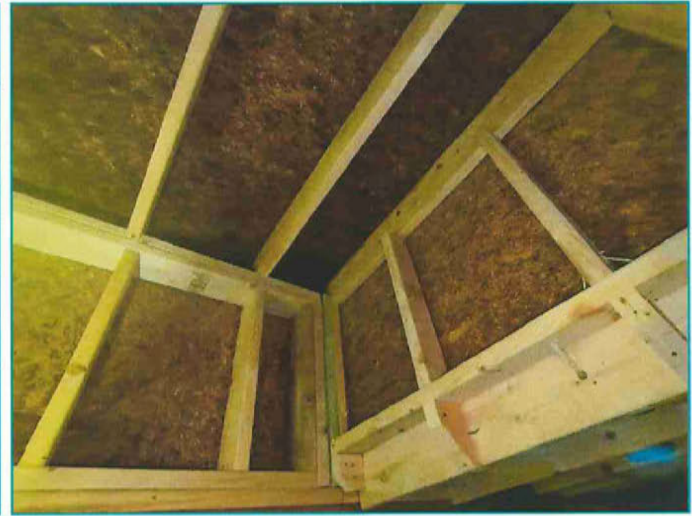
Wet conditions and suspected mold staining at basement rear entry. (outside of living space)
