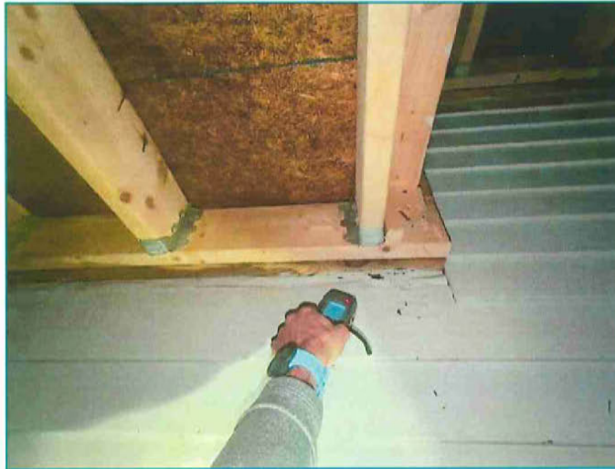
Wet conditions / roof leak at rear basement entry.
