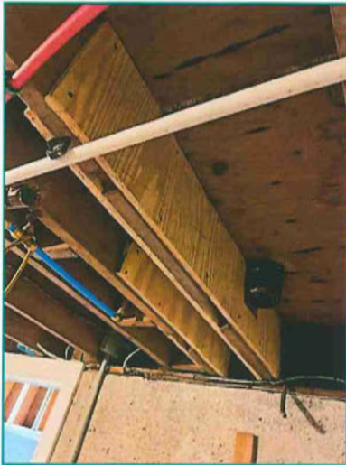
Repairs to previously damaged / notched joists in basement (3/6/2024). Repairs appear to adequately address prior damage.
