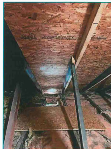
Additional repairs to attic framing (3/6/2024). Roof structure repairs appear to adequately address prior damage.
