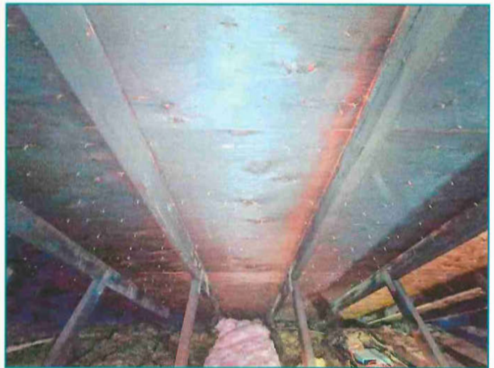
Staining on framing from previous fire. Staining on framing throughout attic tested dry.
