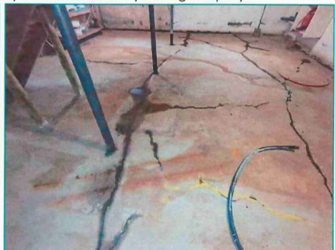
Wet conditions in basement
