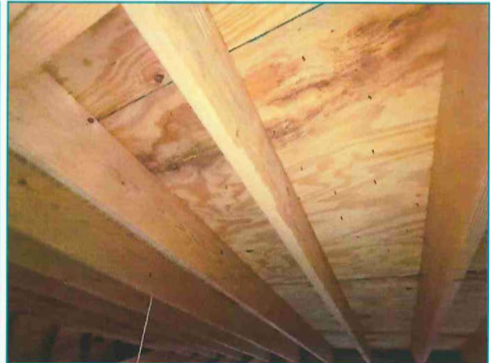
Suspected mold staining at garage ceiling. Area tested dry.
