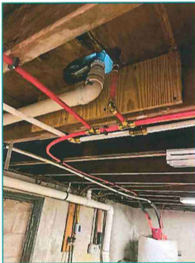
Repairs to previously damaged / notched joists in basement (3/6/2024). Repairs appear to adequately address prior damage.
