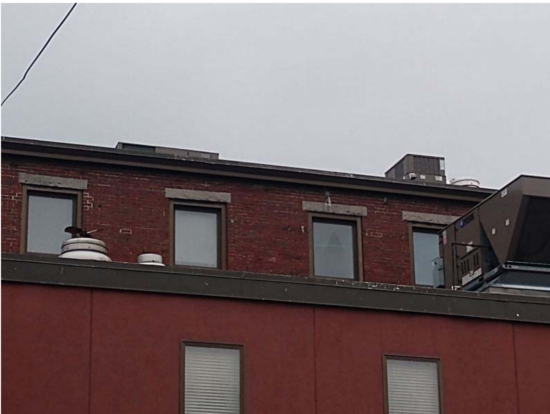
Rear view of Martha's Exchange. Two vent stacks on the left of image are the kettle exhausts. Note that they are well below the roof line.
