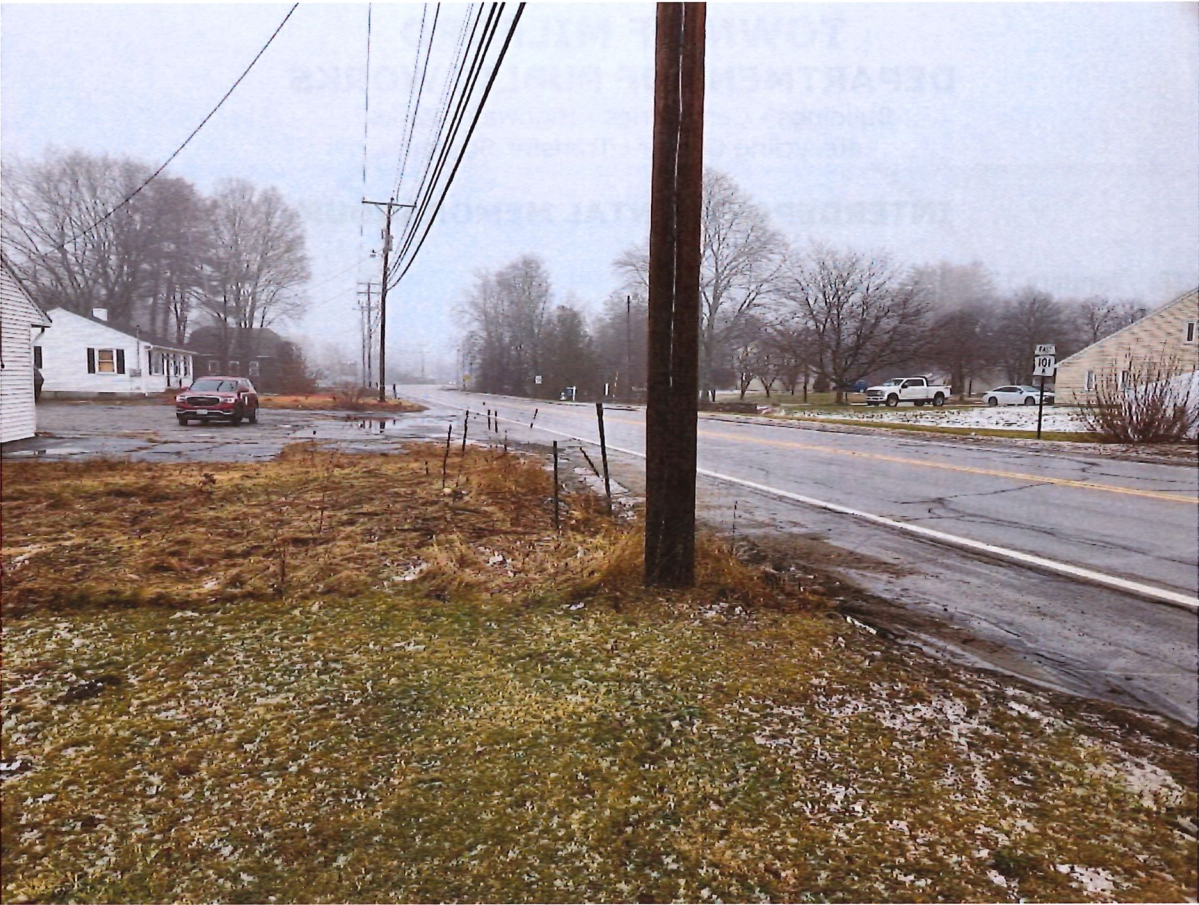
View Easterly along Elm Street at the existing entrance. Puddle along frontage, the inlet to the culvert is at the stake.
