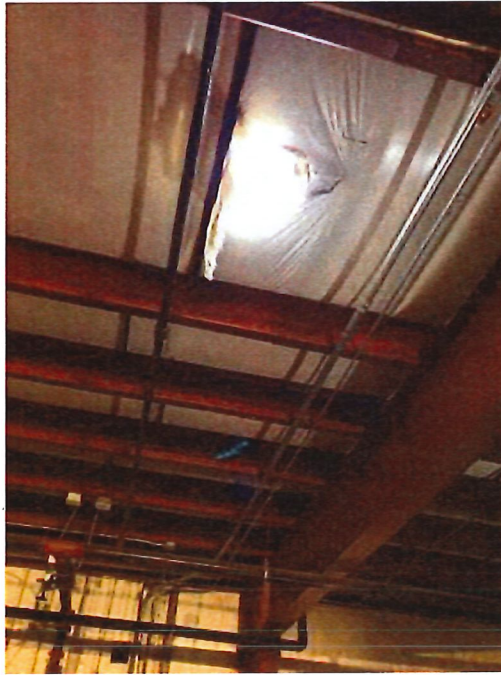
Daylight through hole in insulation, vinyl layer and roof panel
