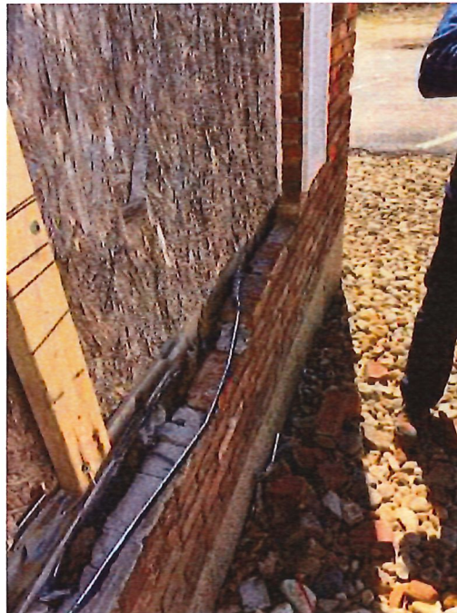
View of failing brick veneer and back up wall below a window opening
