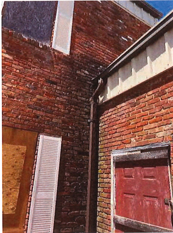
View of brick damage at interior corner
