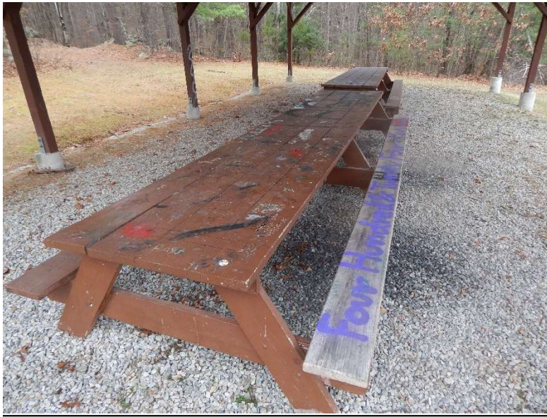
1. Graffiti and spray paint visible on picnic tables in Pavilion
