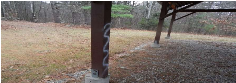
3. White spray paint visible on support timber for Pavilion
