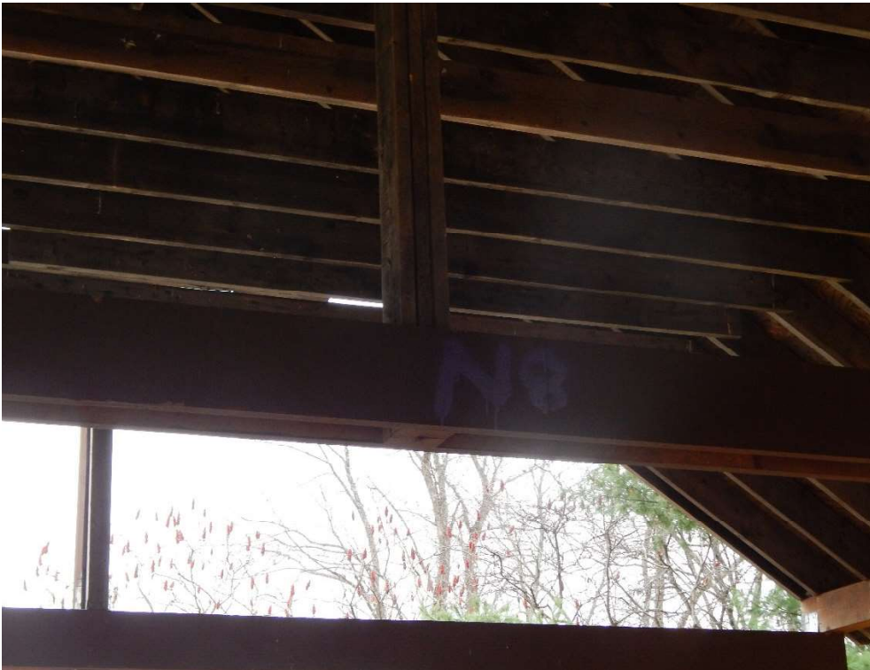
7. Purple spray paint graffiti visible on wooden support beam of roof truss of Pavilion.
