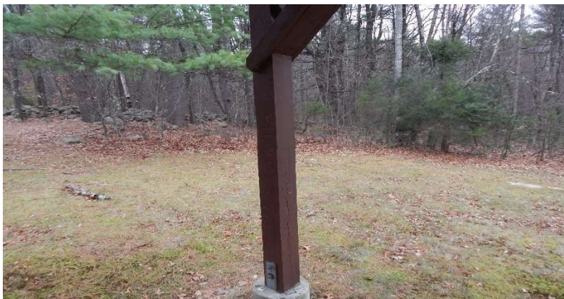
4. Visible graffiti carved into support timber for Pavilion
