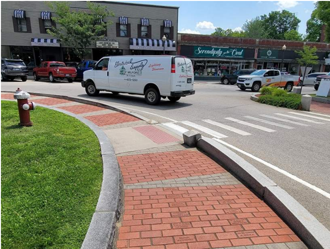
View looking south of the crosswalk from the Oval to the Elm Street median island at the southwest corner of the Oval (Note truck damaged granite)
