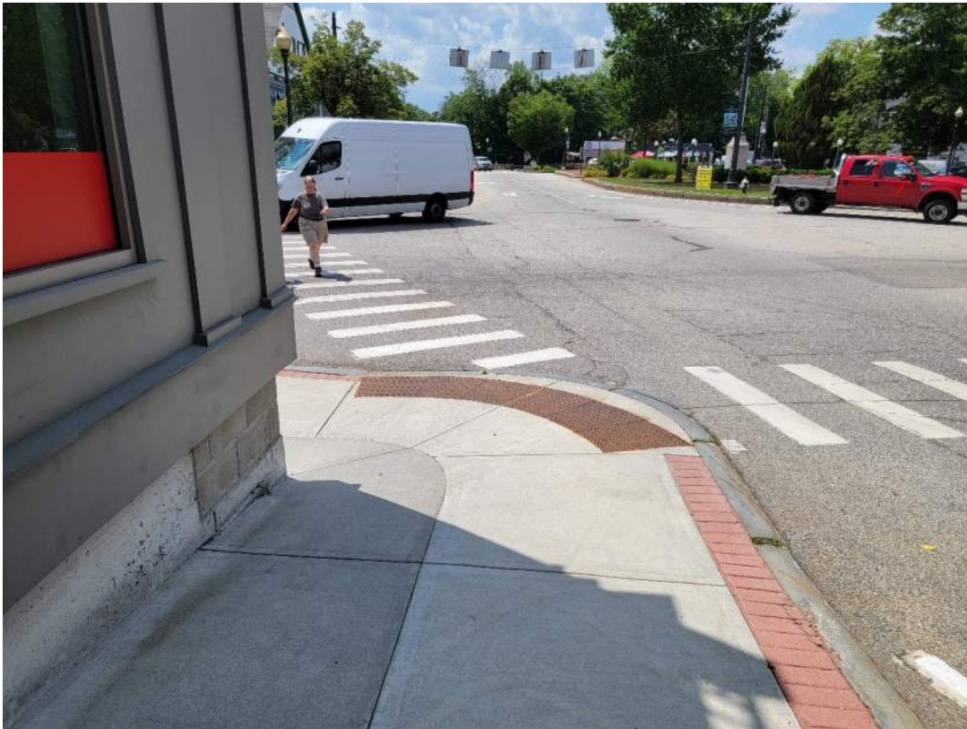
View of existing curb ramp at southeast corner of South Street and Nashua Street, looking west into the Oval
