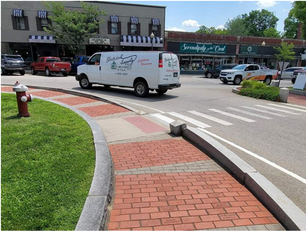
View looking south of the crosswalk from the Oval to the Elm Street median island at the southwest corner of the Oval (Note truck damaged granite)
