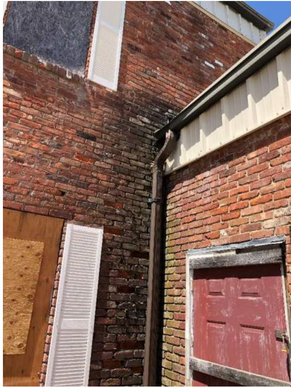
View of brick damage at interior corner
