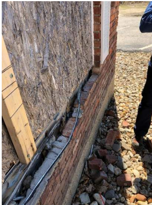
View of failing brick veneer and back up wall below a window opening
