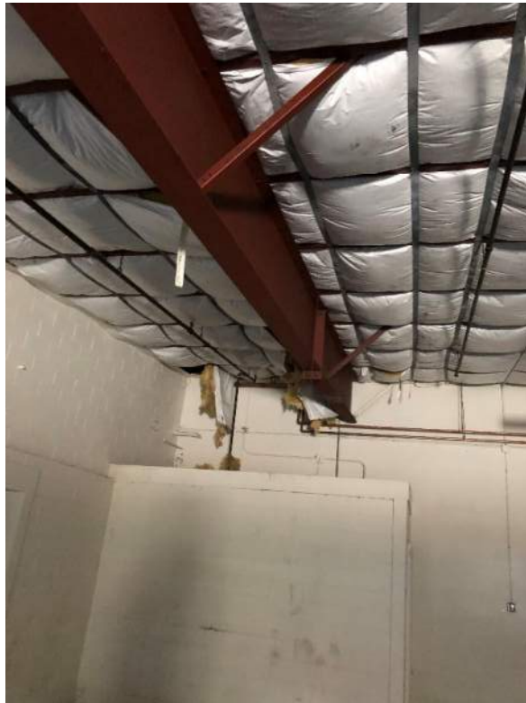
Typical roof insulation with vinyl facing and support strapping
